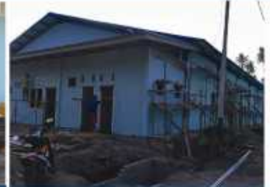
Integrated Coldstorage 200 Ton (PPI Daruba)
